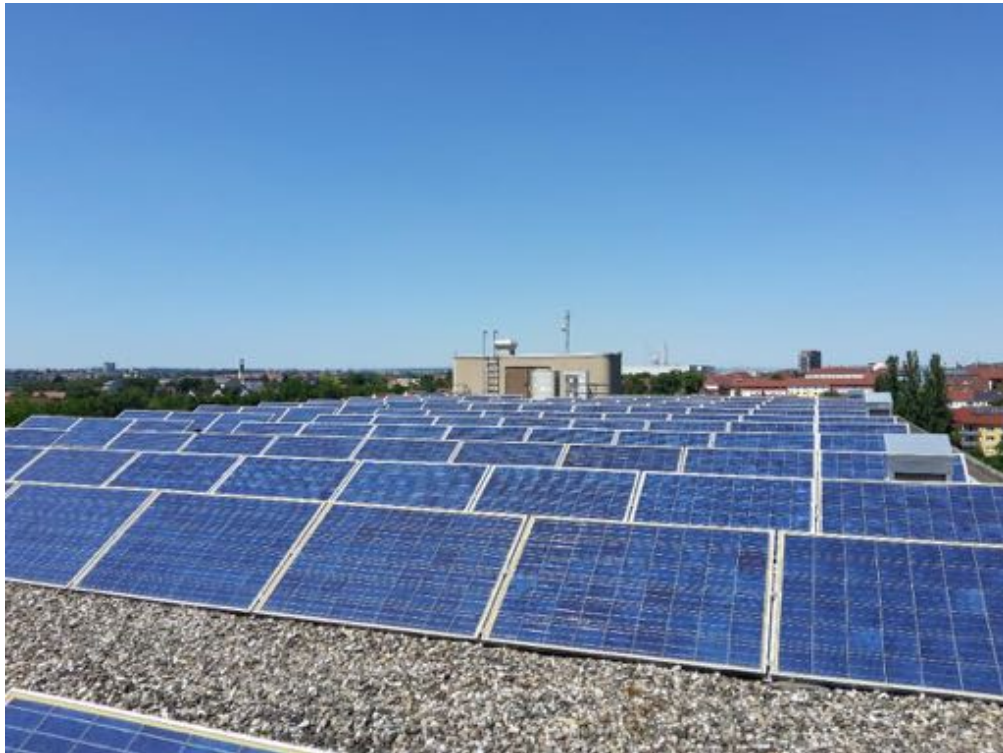
Figure 19: Solar Systems on the Roof of the University.
